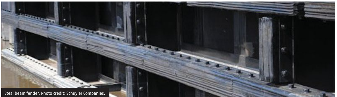
Steel beam fender. Photo credit: Schuyler Companies.
