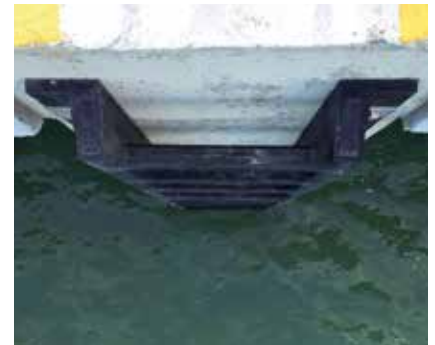
Feed Solid Product Jetty | Johor | Malaysia
